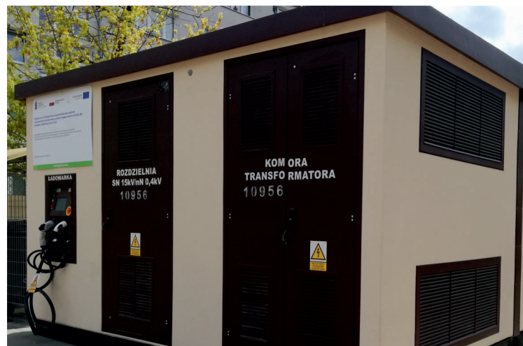
Stacja SPS dla E.ON. (dawniej innogy) E.ON. (formerly innogy) SPS station in Warsaw
